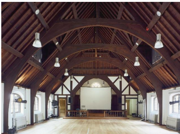
Image 5.23, Retention of quality, the existing roof was deemed worthy of retaining and felt it would not only provide continuity but add to the character of the new use in the building.
