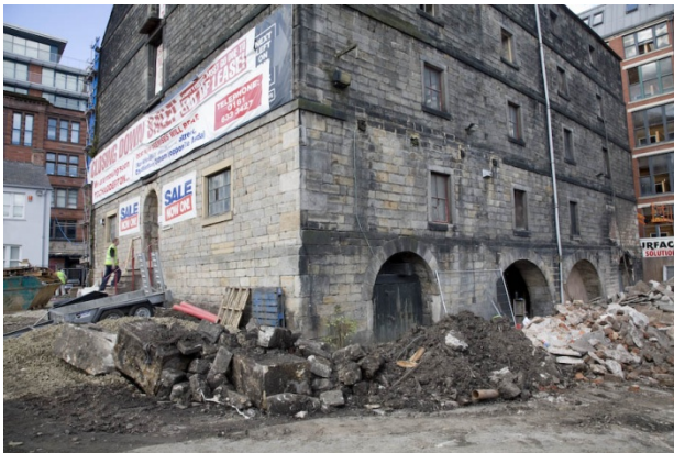
Image 5.26, A view of the existing building. Showing how run down the warehouse has become and the state of decay the area was in before the new use and new interventions were applied.
