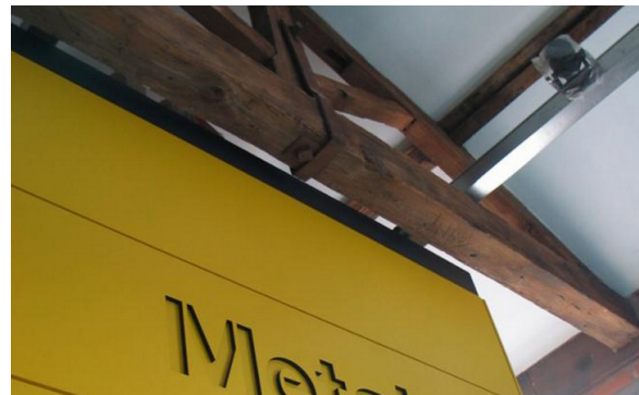
Image 5.6, Edge Hill Galleries, existing roof structure remains intact and the new additions of the 'Metal' workspace does not subtract from the quality as it sits away from the existing.
